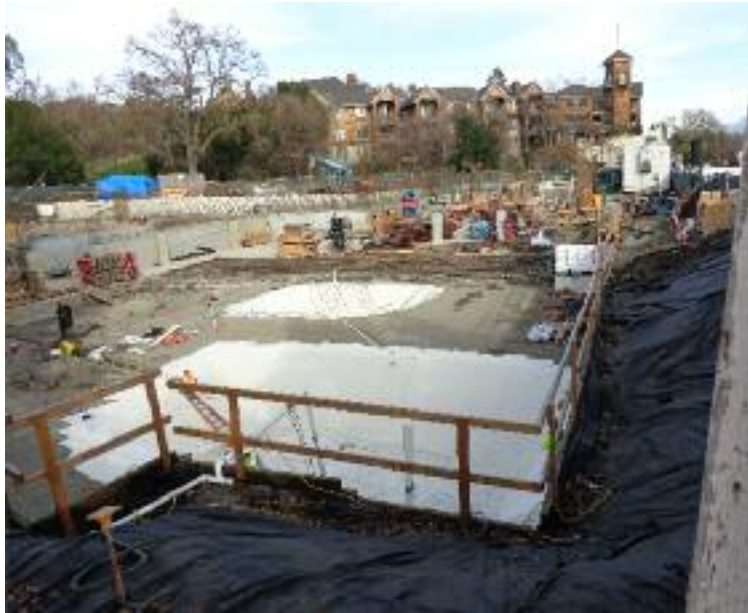
Construction site of the future Towne Center by KB Homes in downtown Lafayette
